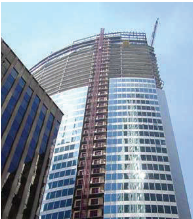
Construction Sector Fireproofing
