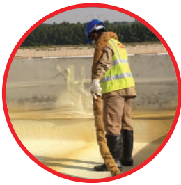
Modern Combo Roofing
